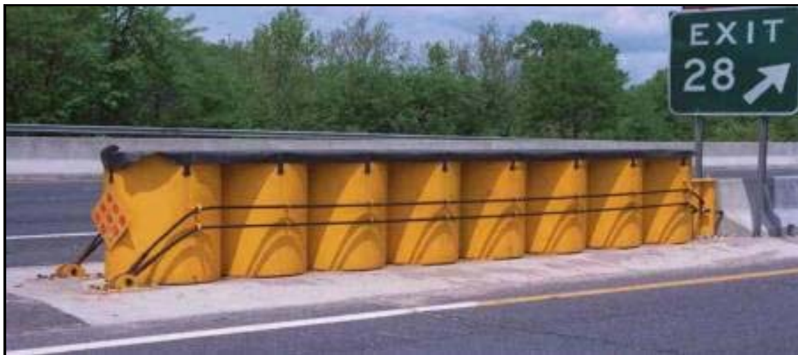
Figure 7. Narrow Connecticut Impact Attenuation System (Photo from CDOT).
